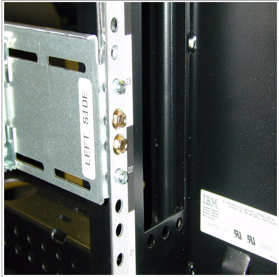
Figure 3-13 Rear rail pin in noted hole location
